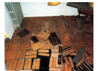
Costly Finishes Damage
