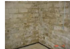
Damp Basement Walls
