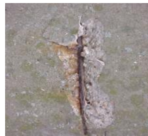
Corrosion of Steel Bars
