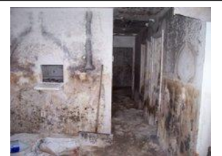
Mildew, Brown spots & Peeling Paint
