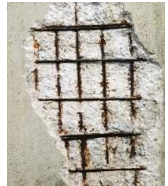
Chloride Penetration attacks steel reinforcement causing corrosion, and results in concrete cracking and spalling.
