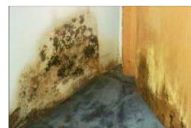
Mold On Walls
